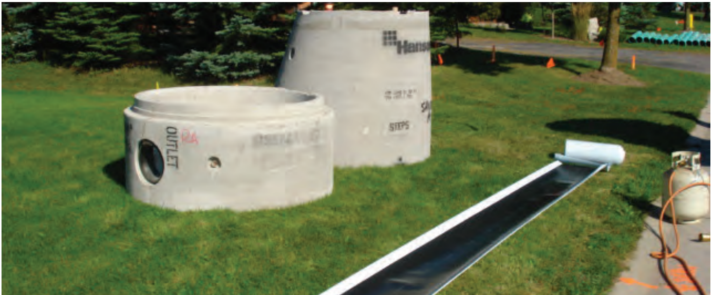
Figure 8 – Riser-Wrap Used to Seal New Maintenance Hole in the Township of King to Prevent Ground Water Infiltration.
