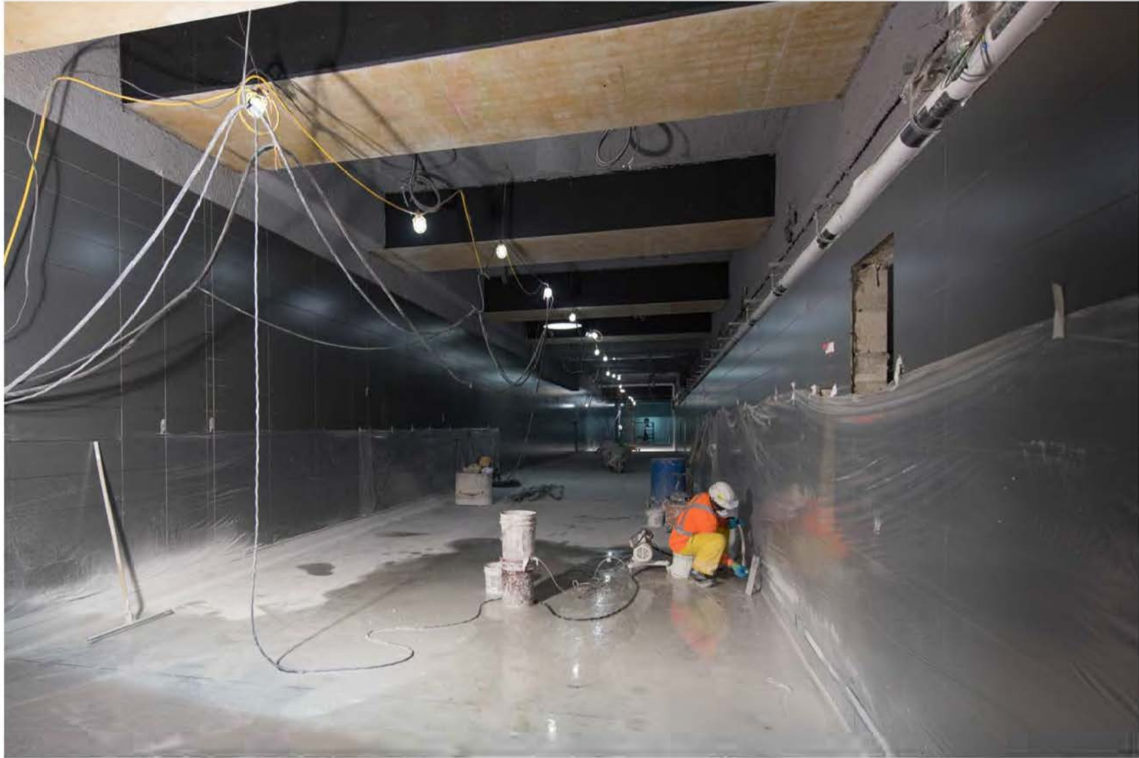
Vaughan Metropolitan Centre Station Tile finishing work underway in the pedestrian tunnel connection to YRT bus terminal
