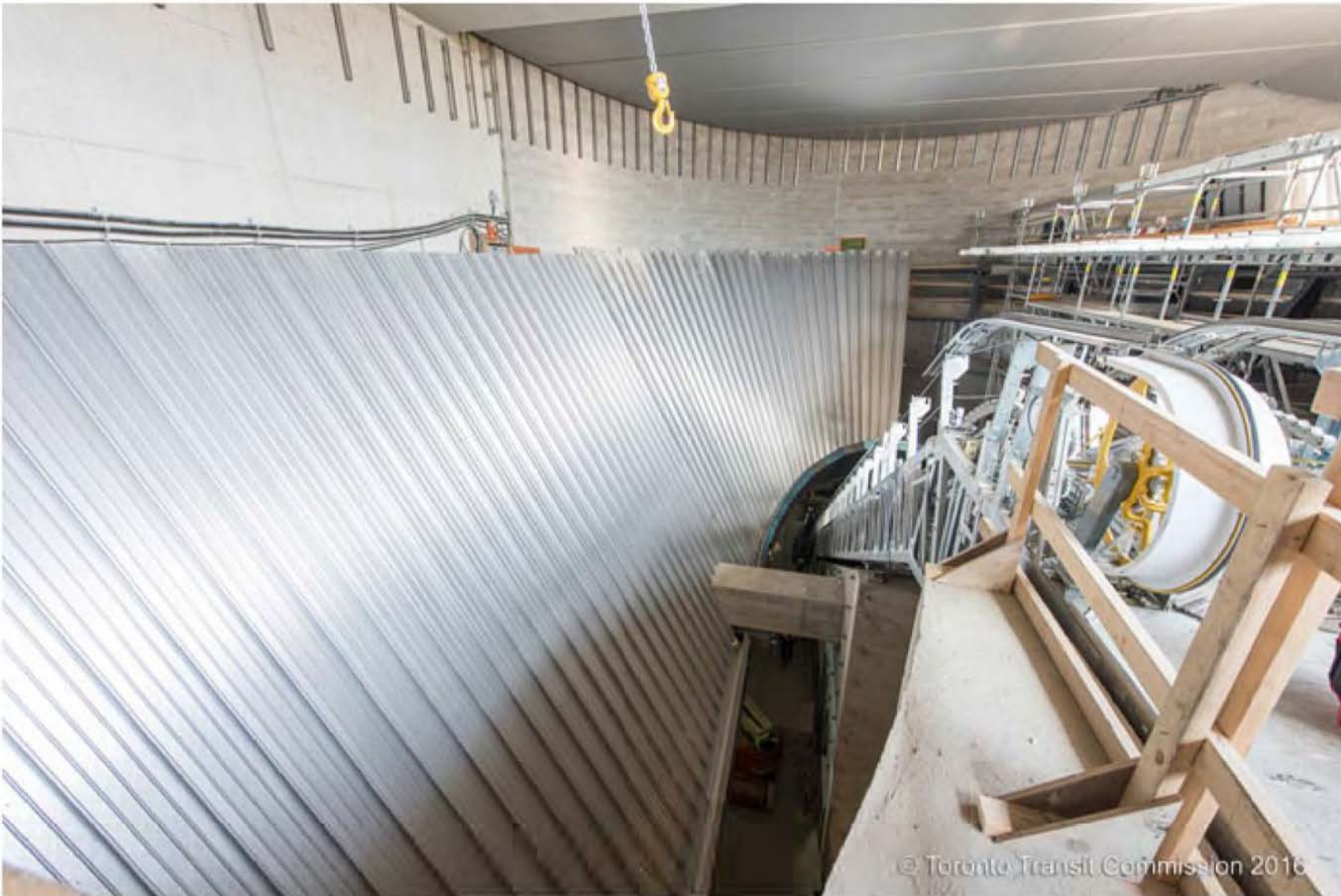
Highway 407 Station View down side of escalator connecting concourse to platform – velodrome cladding in progress
