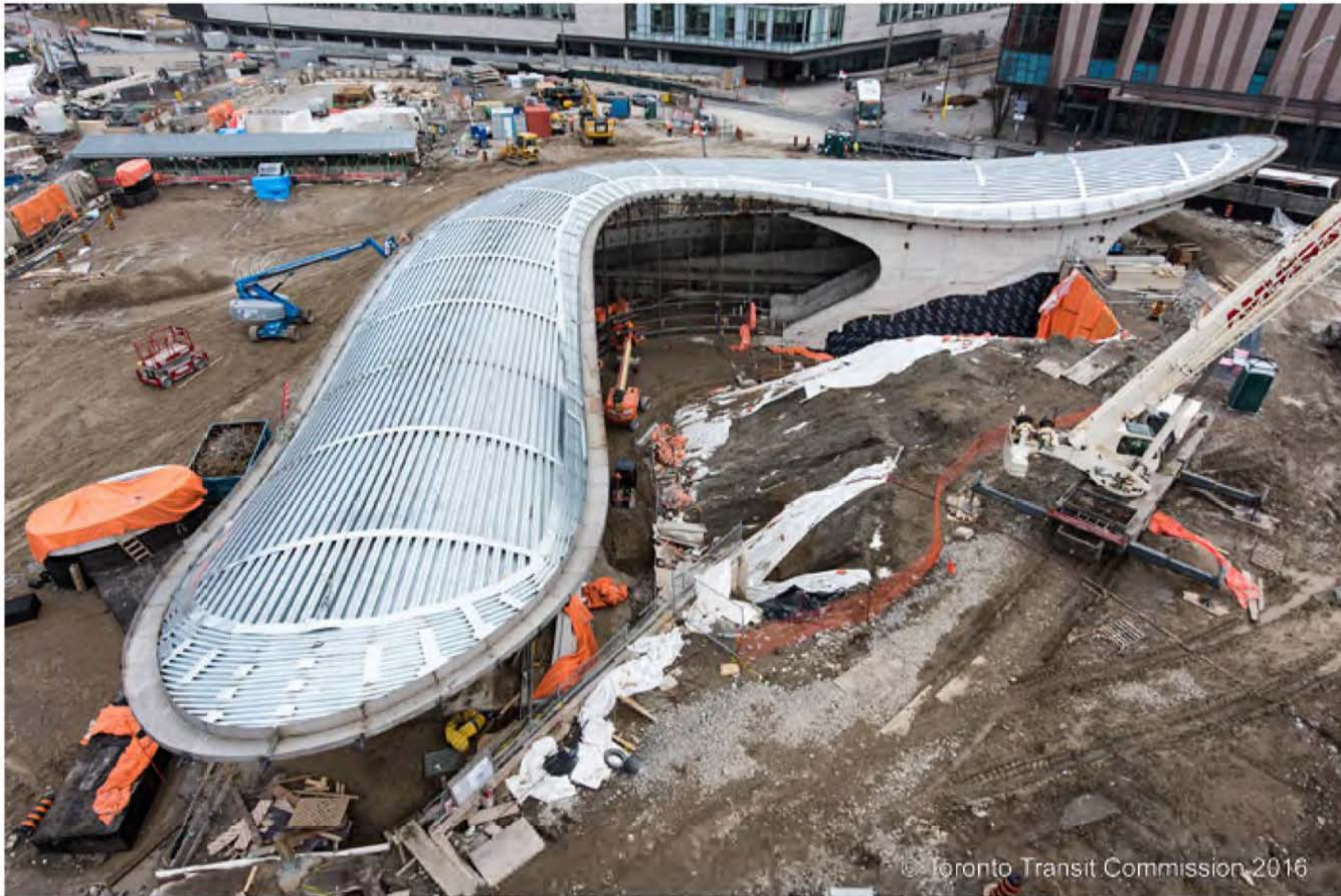
York University Station Station entrance structure view from Kaneff Tower First layers of roof cladding complete
