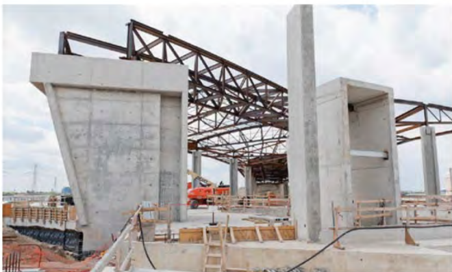
The structural steel roof trusses on top of the bus terminal. – May 22, 2015
