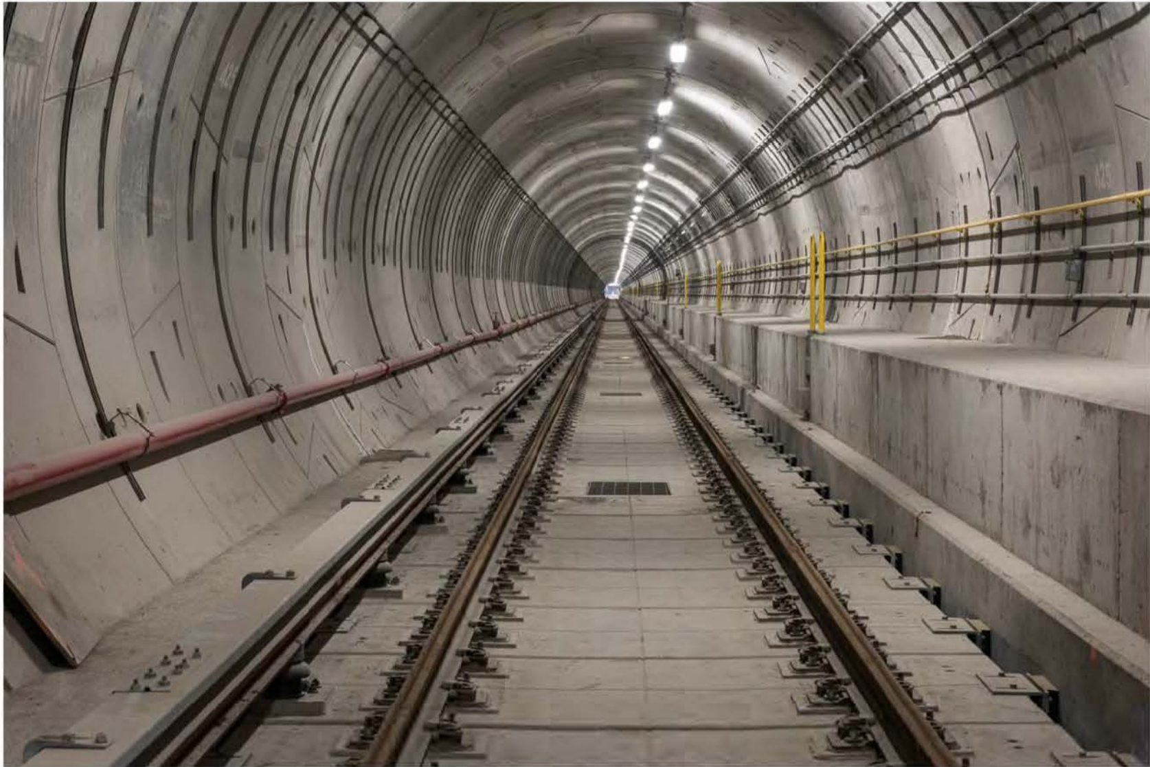
York University Station Tunnel between York University and Pioneer Village stations Tunnel equipping in progress
