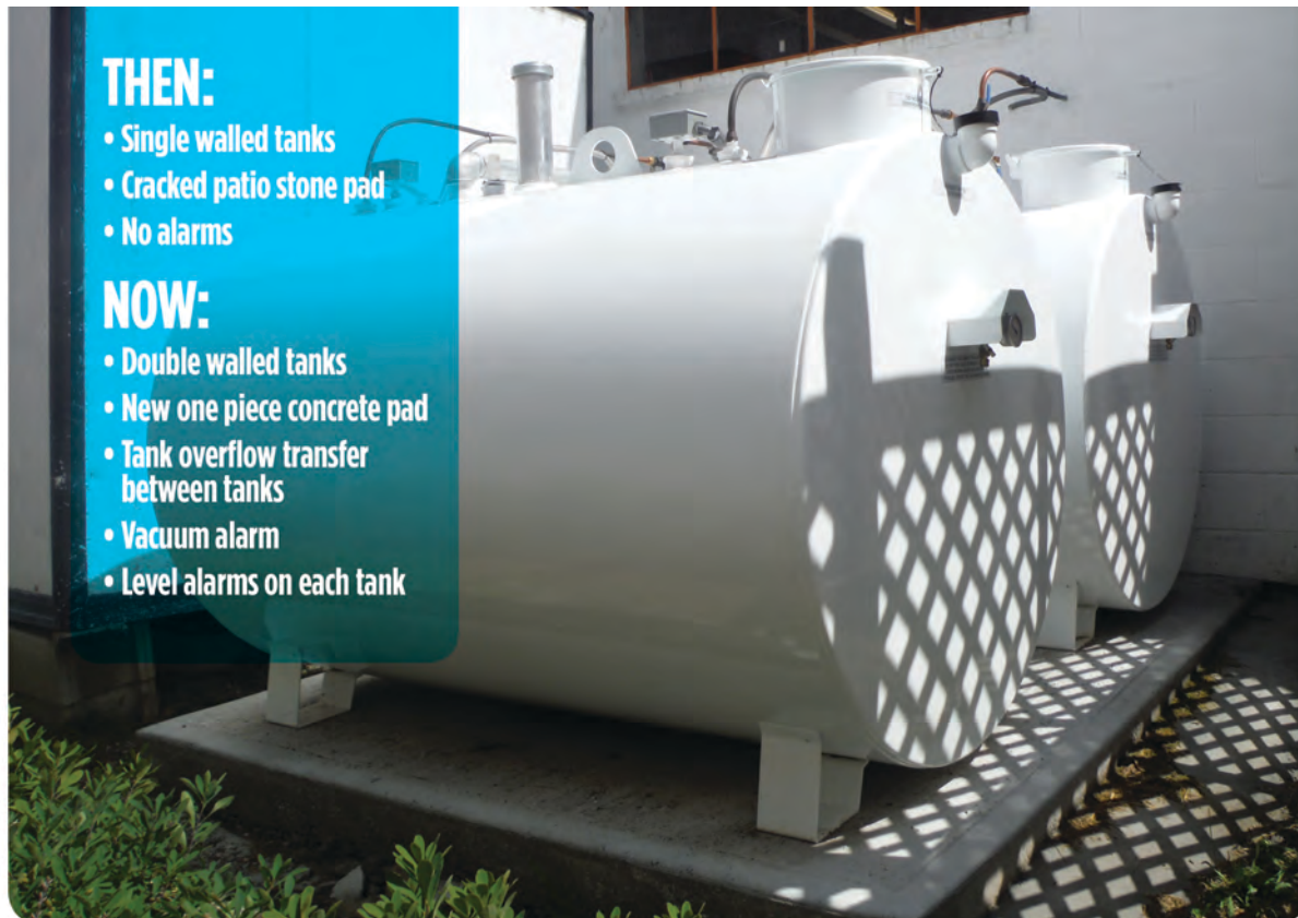
Figure 14 – New Tank System With Improved Risk Management Measures
