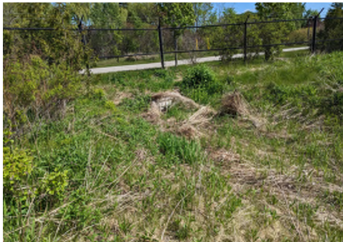
PHOTO 9: View of a culvert on the southeastern portion of the Site, to the south of the previously identified culvert, facing northeast.
