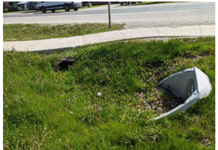
PHOTO 10: View of culverts to the east of the Site, at Highway 27, facing east.
