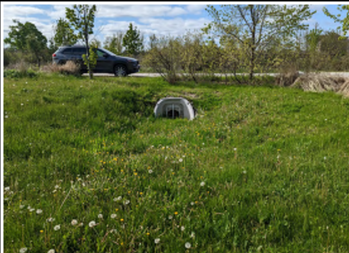
PHOTO 7: View of a culvert on the eastern portion of the Site, facing south.
