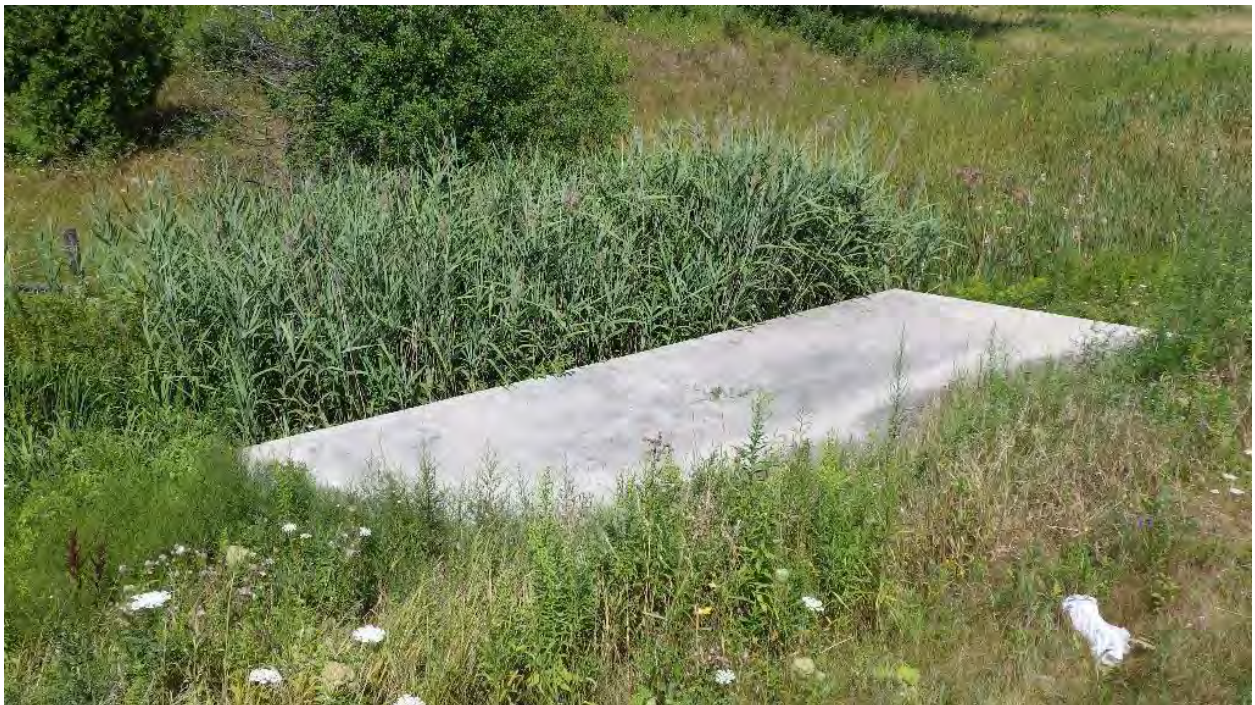
Photo 10: Fisheries Site 2 - Dense Phragmites at culvert inlet upstream of Teston Road
