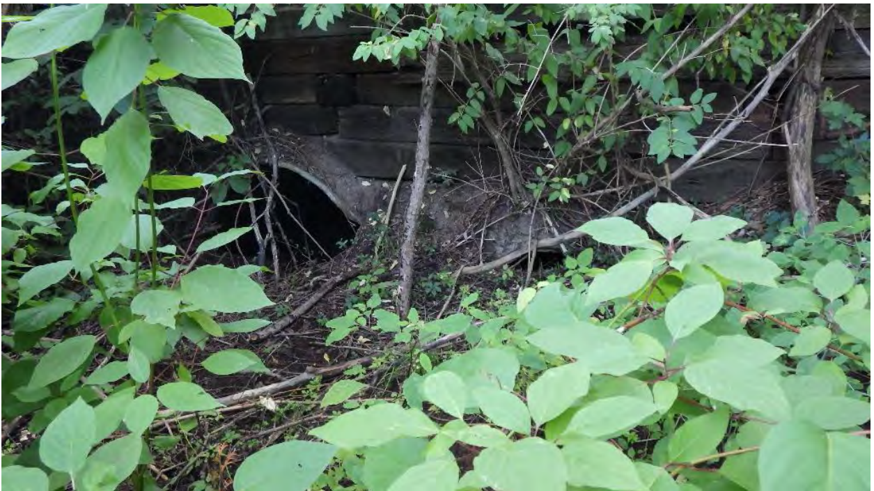
Photo 14: Fisheries Site 2 - Pedestrian bridge on private property with blocked CSP culverts
