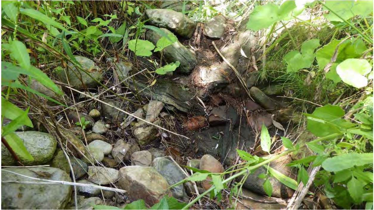
Photo 17: Fisheries Site 3 - Dry cobble channel and landscape fabric upstream of the culvert inlet
