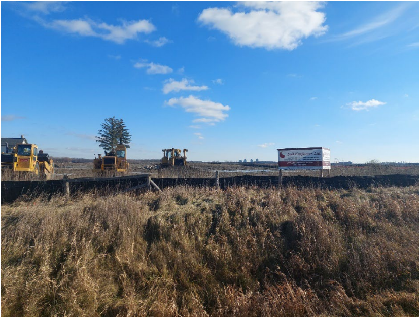
Plate 22: View of construction on the eastern side of Kennedy Road, looking east.
