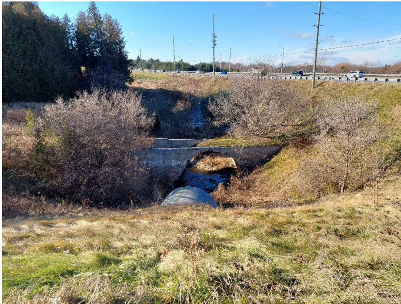
Plate 9: View of the corrugated metal culvert in the foreground and the remains of the former bridge for Warden Avenue in the middle ground, looking west.
