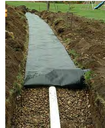
Geotextile being used to prevent fines from entering the trench above. Source: https://wiki.sustainabletechnologies.ca/images/f/f5/North_Dakota_State_U_infiltration_trench.jpg
